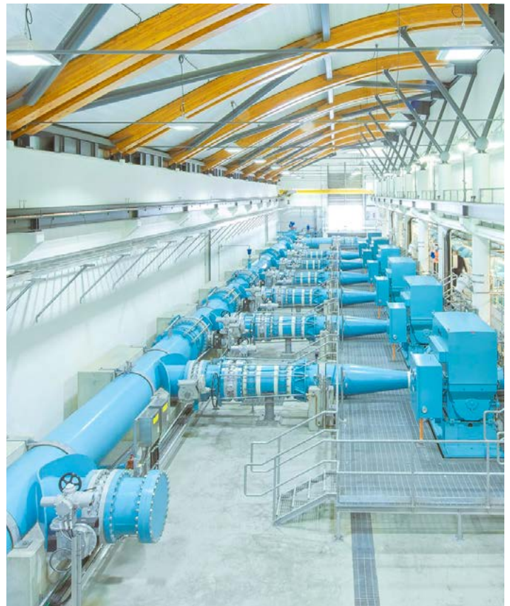
Barnston-Maple Ridge Pump Station.
