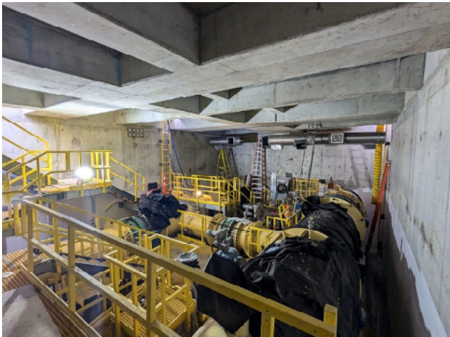
Figure 18: Kennedy Newton Water Main – Installation of Piping and Valves within the Large Underground Valve Chamber
