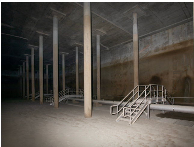
Figure 14: a. Inside Clayton Reservoir – prior to cleaning April 2023 b. Inside Clayton Reservoir – post cleaning February 2024
