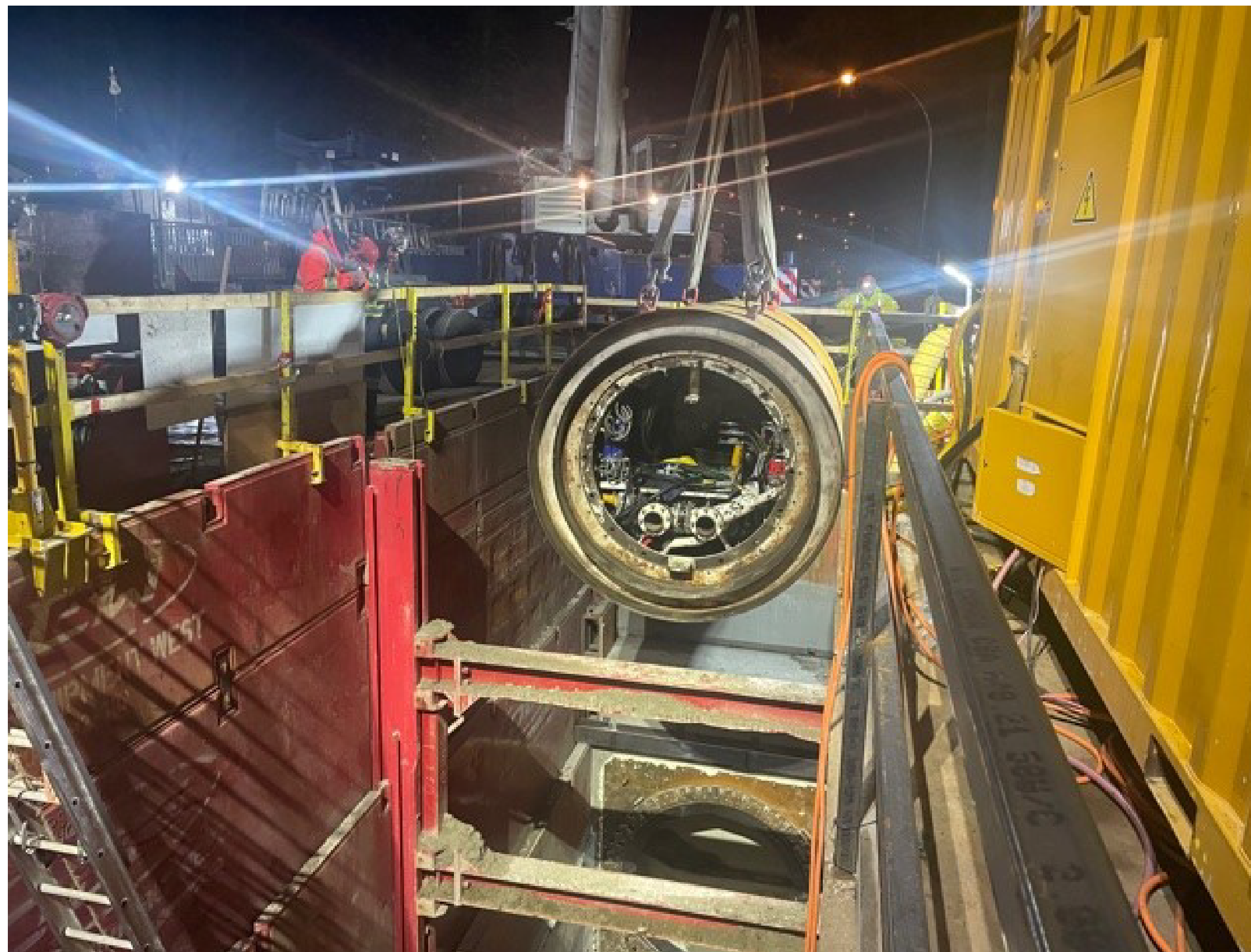
Tunnel boring machine used to excavate the tunnel for the Kennedy Newton Water Main South Section project. A similar machine may be used to excavate a tunnel for the Kingsway crossing section.
