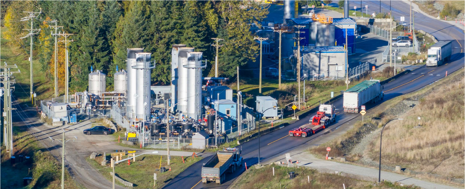
Vancouver Landfill flare station
