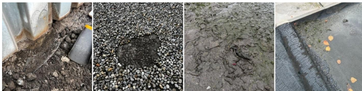
Figure 16. Accumulated material on roofs, from left to right Waste-to-Energy Facility roof, Garibaldi Glass roof, Wigg roof, and Wigg Surrey roof.
