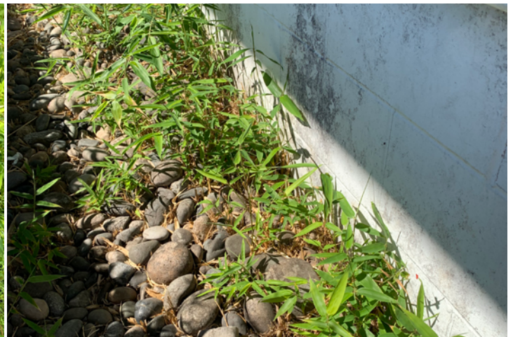
Running bamboo growing next to a foundation CREDIT: ISCMV
