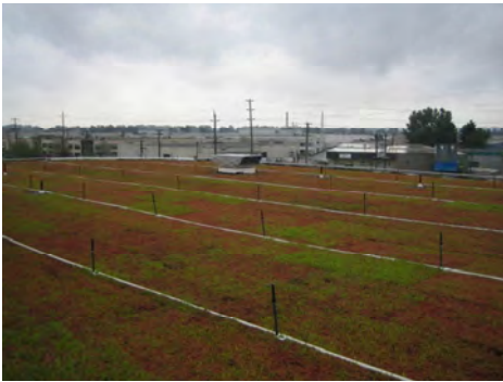
Extensive Green Roof on a warehouse in Port Coquitlam, BC.
