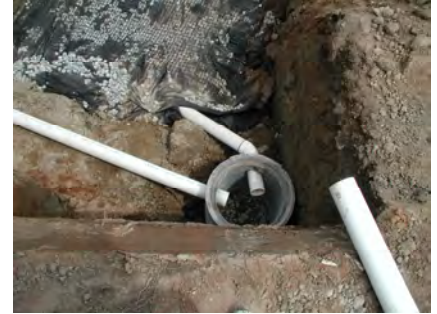
Single family lot infiltration trench being installed in East Clayton development, Surrey, BC.
