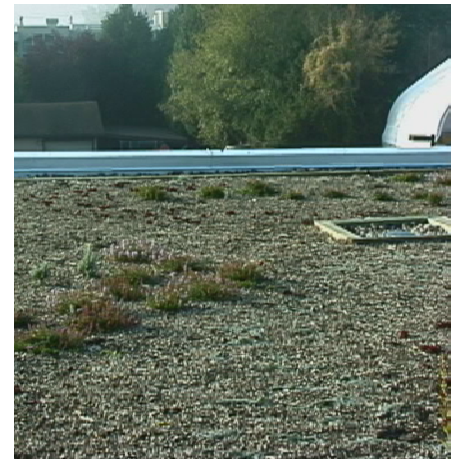
Newly planted extensive green roof showing plant-free zones at drain and edges – White Rock Operations Building
