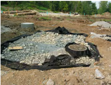
Infiltration trench with catch basin inlet at Silver Maples Subdivision in Maple Ridge, prior to surface cover with filter cloth and growing medium.
