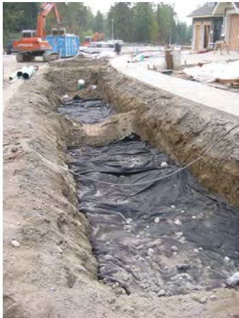
Same infiltration trench as above, before backfill, showing filter cloth wrap, and showing trench dam of native material between infiltration trench 'cells'.
