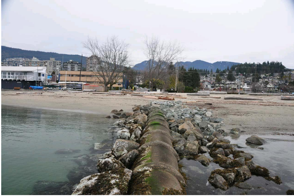
Photo A5 - Piped system outfall (Ambleside, West Vancouver, BC).
