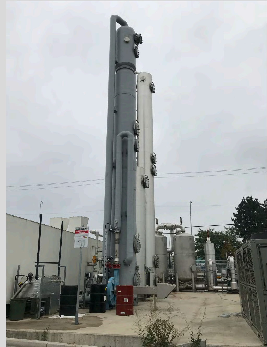
Biogas upgrade system at Surrey Biofuel Facility
