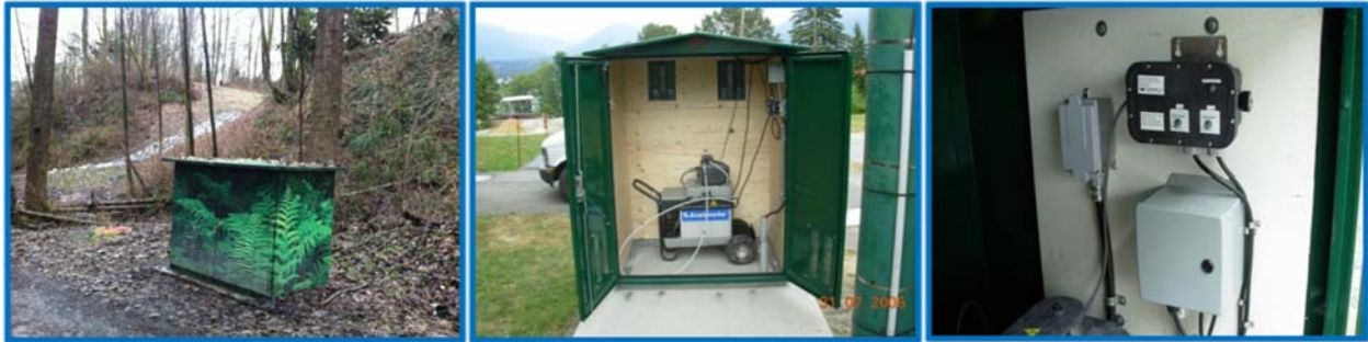
FIGURE 10.3 CSO INFRASTRUCTURE: SAMPLING KIOSK (LEFT), KIOSK WITH AUTOSAMPLER (CENTER), SAMPLER COMMUNICATION ELECTRONICS (RIGHT)
