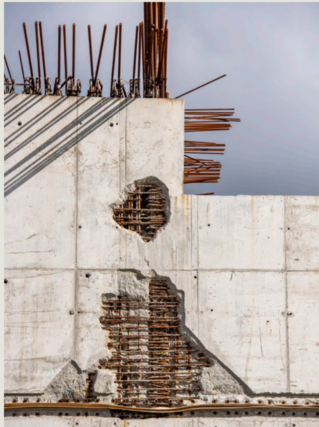
Example of concrete requiring repair
