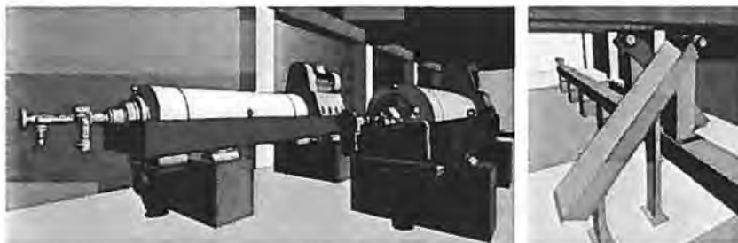
(left) View of centrifuge in the Dewatering Building
