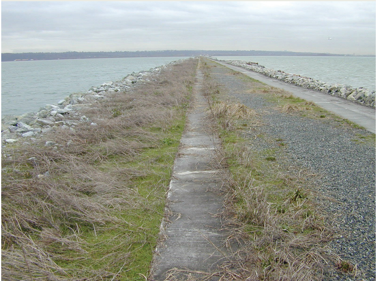
Caption: The view from the Iona Jetty looking north towards the plant
