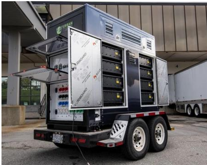
The Urban Power Source battery generator is the largest available in the Metro Vancouver region. Credit: MBSE Canada.
