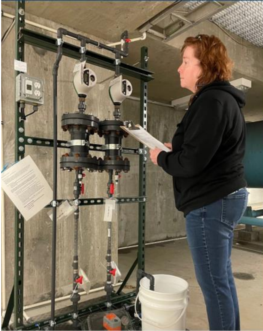
Field Station Installation
