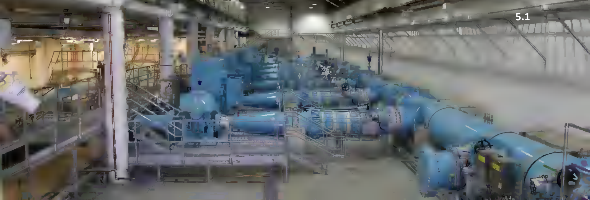
Barnston Maple Ridge Pump Station
