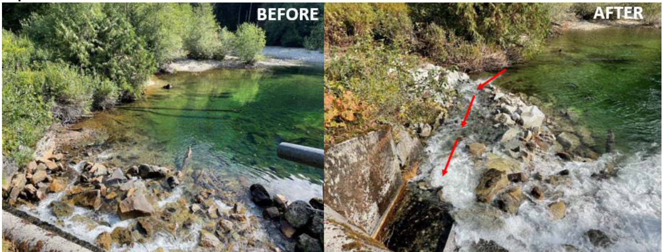
Image 2: Fish passage improvements at the Enchantment Creek bridge crossing in the upper Capilano Watershed.
