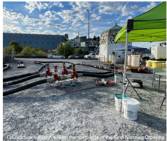
Disinfection injection site on the north side of the First Narrows Crossing
