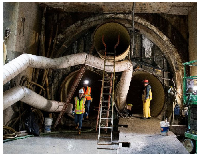
Three water mains inside tunnel
