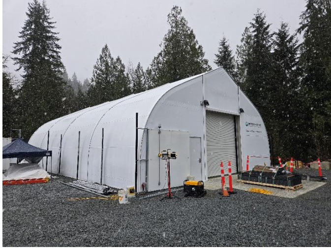
Treatment pilot test plant exterior
