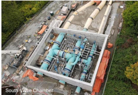
South Valve Chamber
