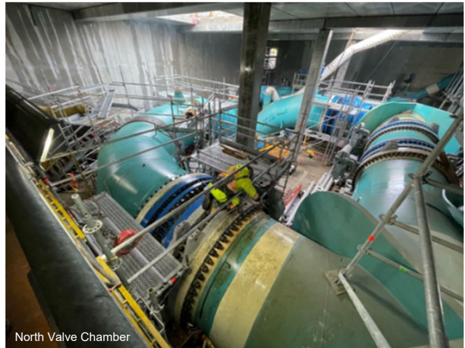
North Valve Chamber
