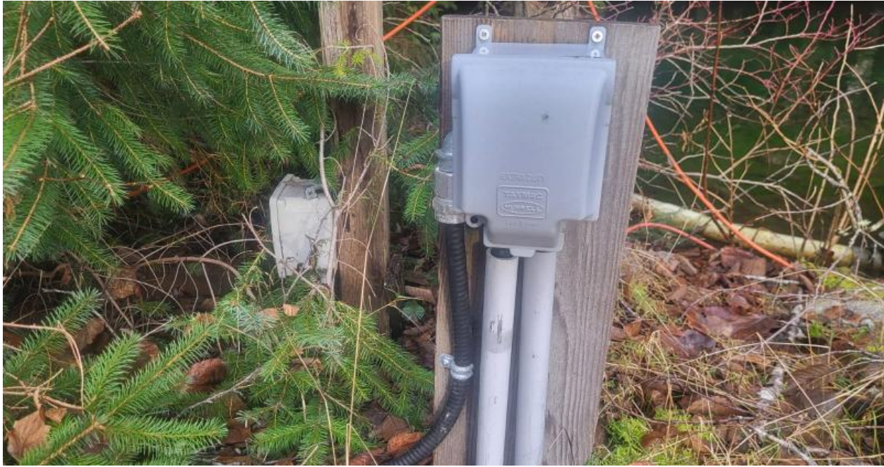
FIGURE 25 EXTERNAL ELECTRICAL BOX CONNECTIONS FOR THE SITE
