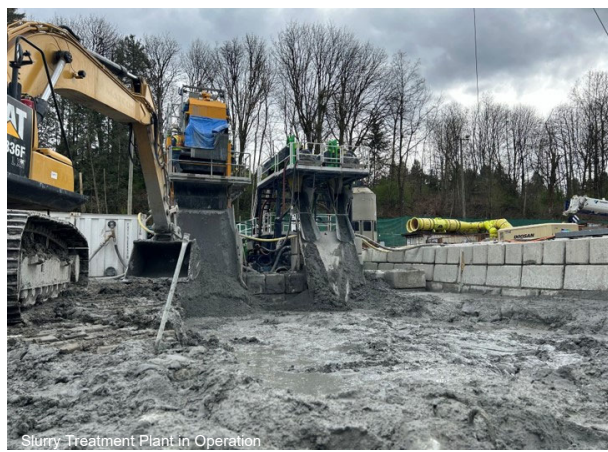
Slurry Treatment Plant in Operation
