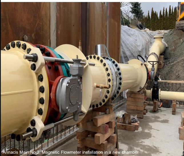
Annacis Main No.2. Magnetic Flowmeter installation in a new chamber
