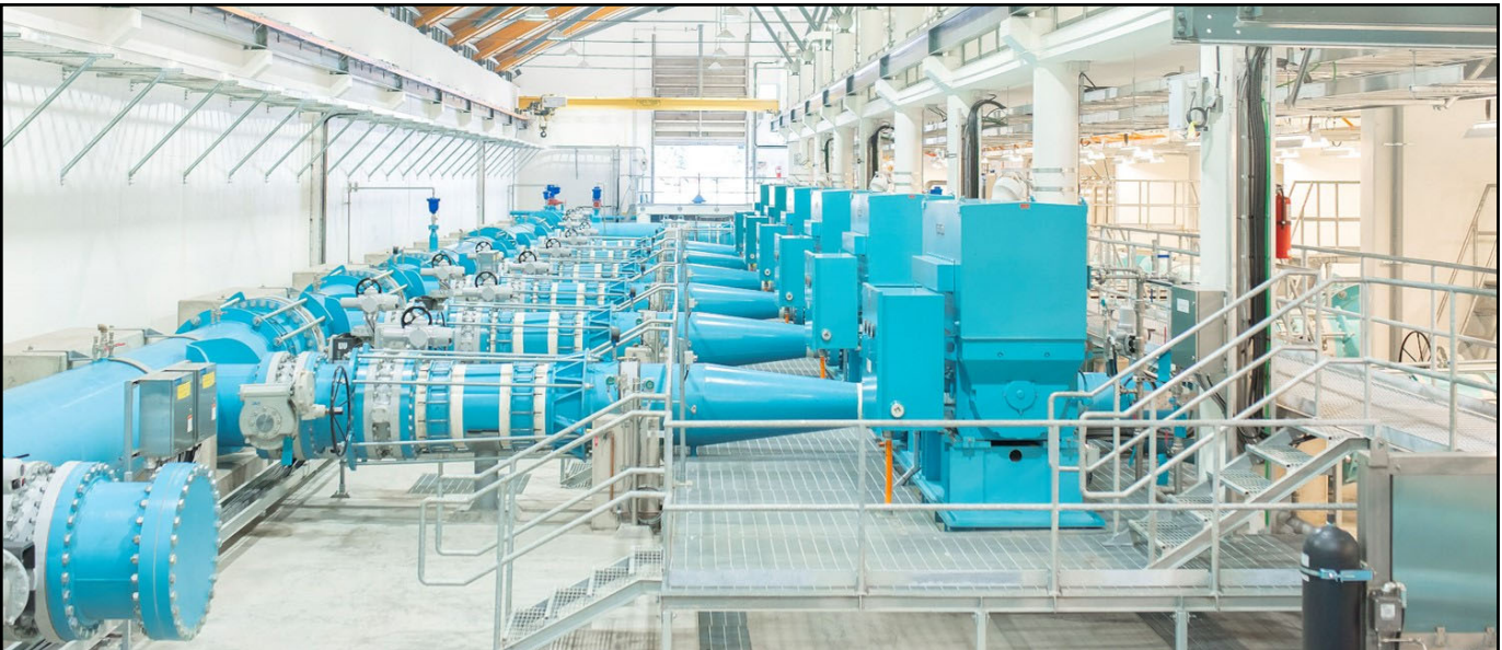
Barnston Maple Ridge Pump Station
