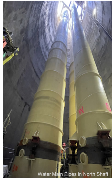
Water Main Pipes in North Shaft
