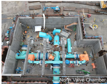
North Valve Chamber
