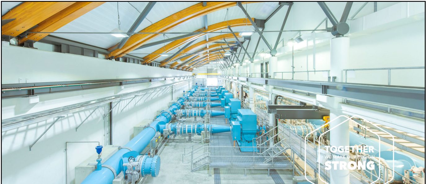
Barnston Maple Ridge Pump Station
