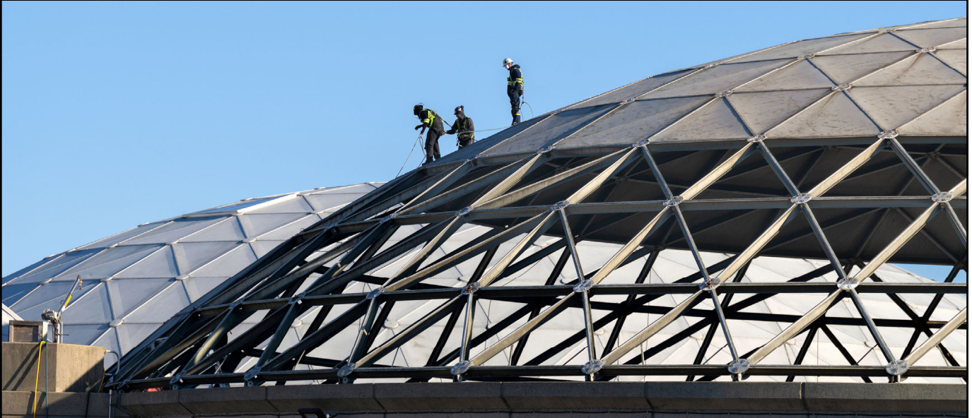
A crew works on the installation of the new trickling filter domes at Annasis Island Wastewater Treatment Plant
