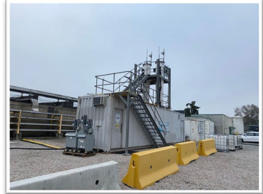
Aerobic Granular Sludge Pilot
