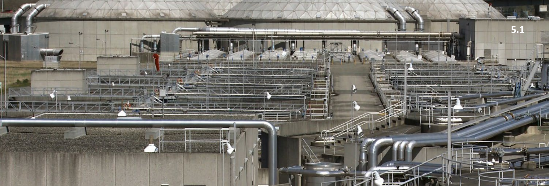
Annacis Island Wastewater Treatment Plant
