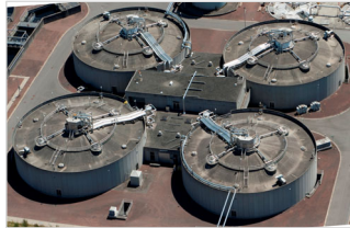
Annacis WWTP Digesters
