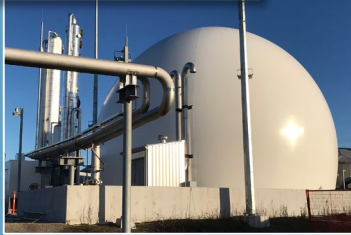
Lulu Island WWTP RNG Facility, Richmond
