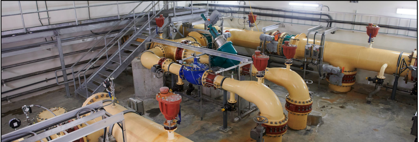
Clayton Reservoir Valve Chamber
