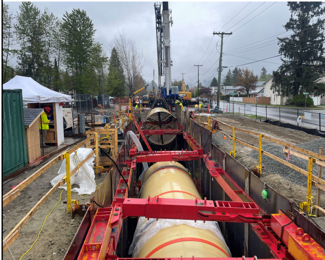
Robson to Guildford Section – 3.2m diameter steel pipe installation at Town Centre Park
