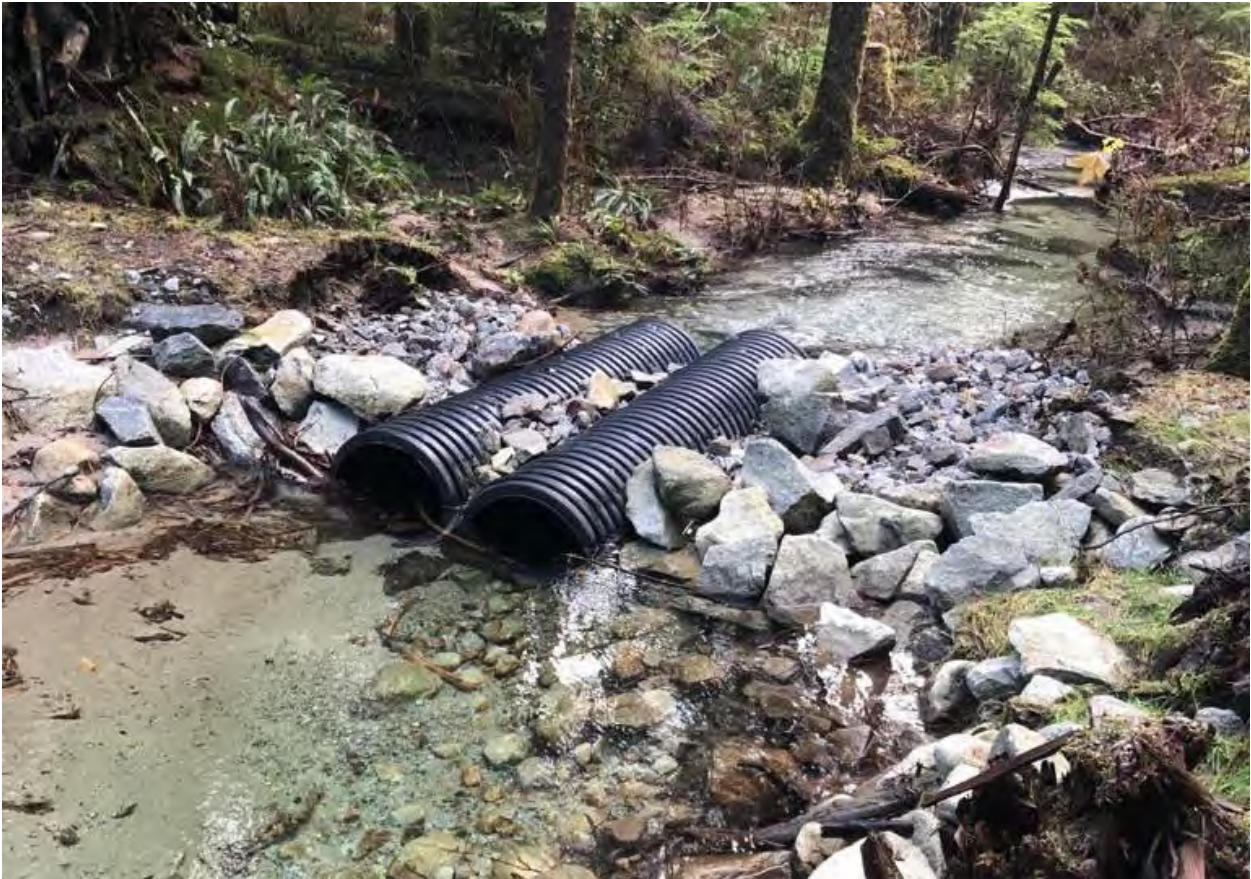
FIGURE 3 SETTLING POND BERM DAMAGE AT JUNIOR CREEK IN NOVEMBER 2023
