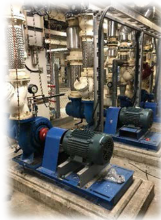
Additional Heating Reservoir Supply Digester Load Pumps to meet future capacity
