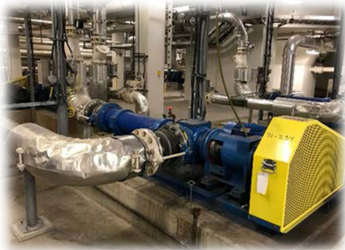
Additional Mixed Sludge Feed Pumps to improve redundancy and meet future capacity
