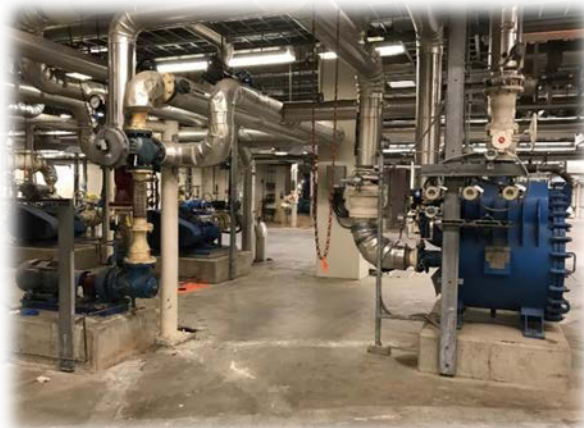
Additional Circulating Sludge/ Heating Reservoir Supply Heat Exchangers with associated Hot Water Circulation Pumps and Digested Sludge Circulation Pumps to meet future capacity
