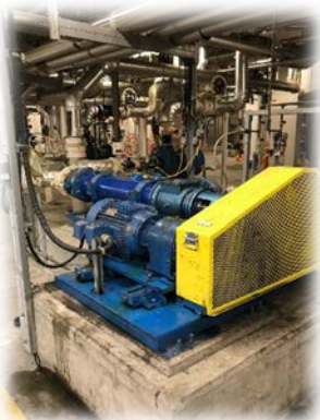
Additional Digested Sludge Withdrawal Pumps to improve redundancy
