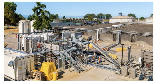
Pilot plant completed Pilot plant
