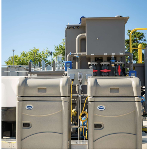
Pilot plant cloth media filters
