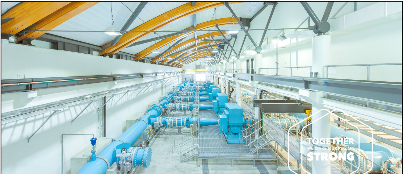
Barnston Maple Ridge Pump Station
