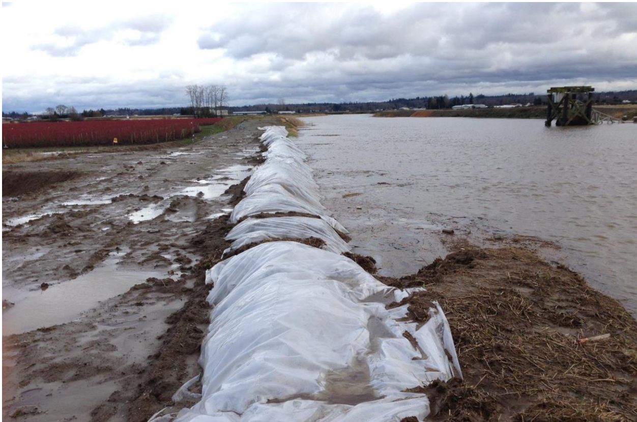
High water protection efforts along the Nicomekl River, Surrey.
