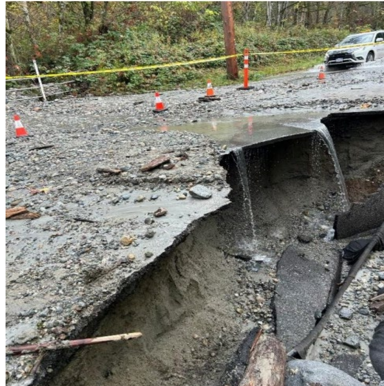
Pipeline Rd Washout
