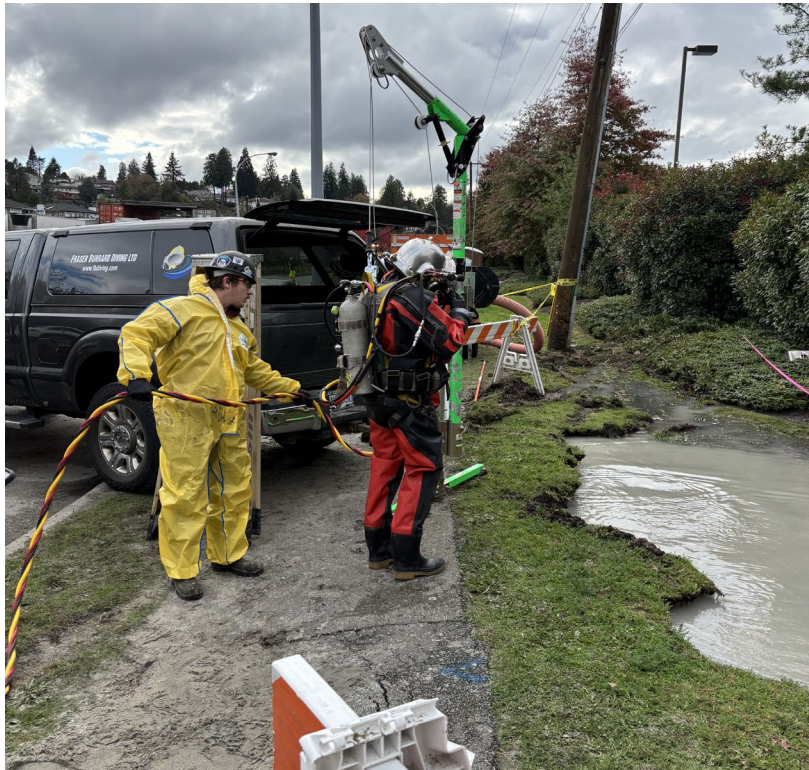
Sewer Break, North Surrey
