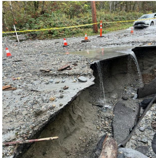
Pipeline Rd Washout
