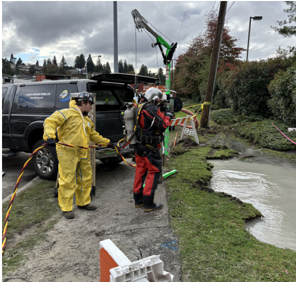
Sewer Break, North Surrey
