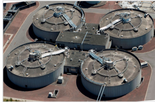
Annacis WWTP Digesters
