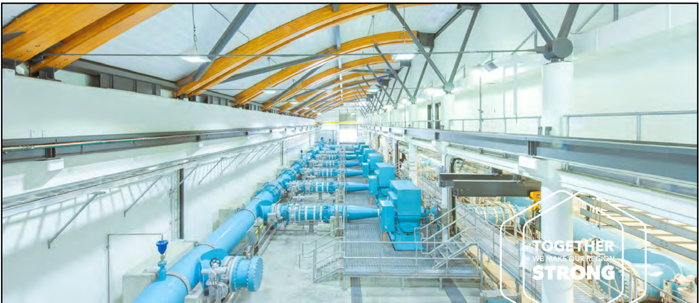
Barnston Maple Ridge Pump Station
